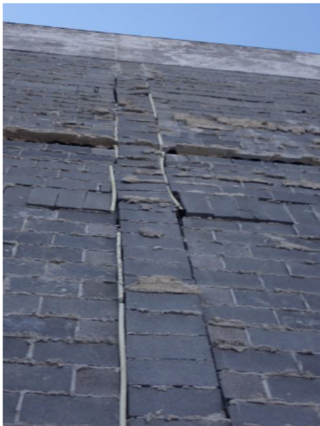
Figure 3. Misaligned and unsupported stack bonded CMU.
