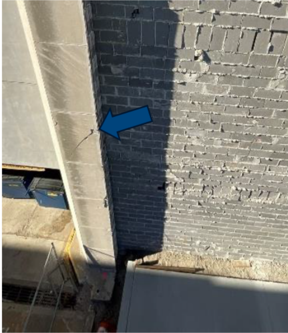
Figure 7. Large crack in limestone panel due to impact damage.
