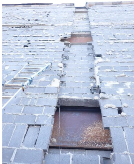
Figure 4. Voids of varying sizes in the east wall.
