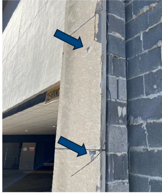
Figure 8. Locally damaged limestone panels.
