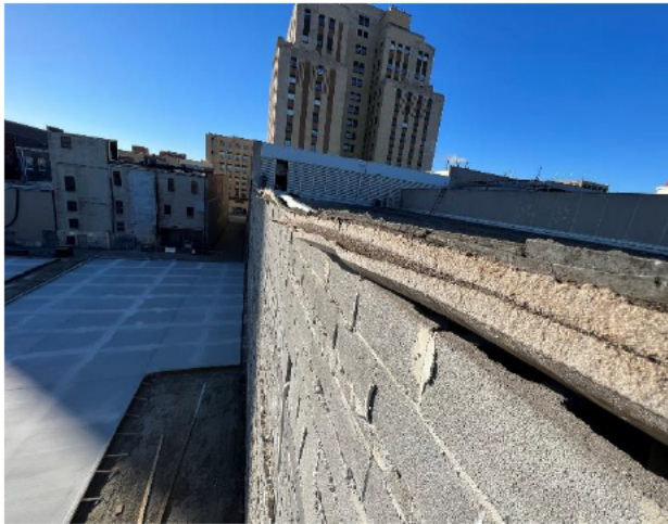
Figure 5. Detached and damaged coping along east elevation.
